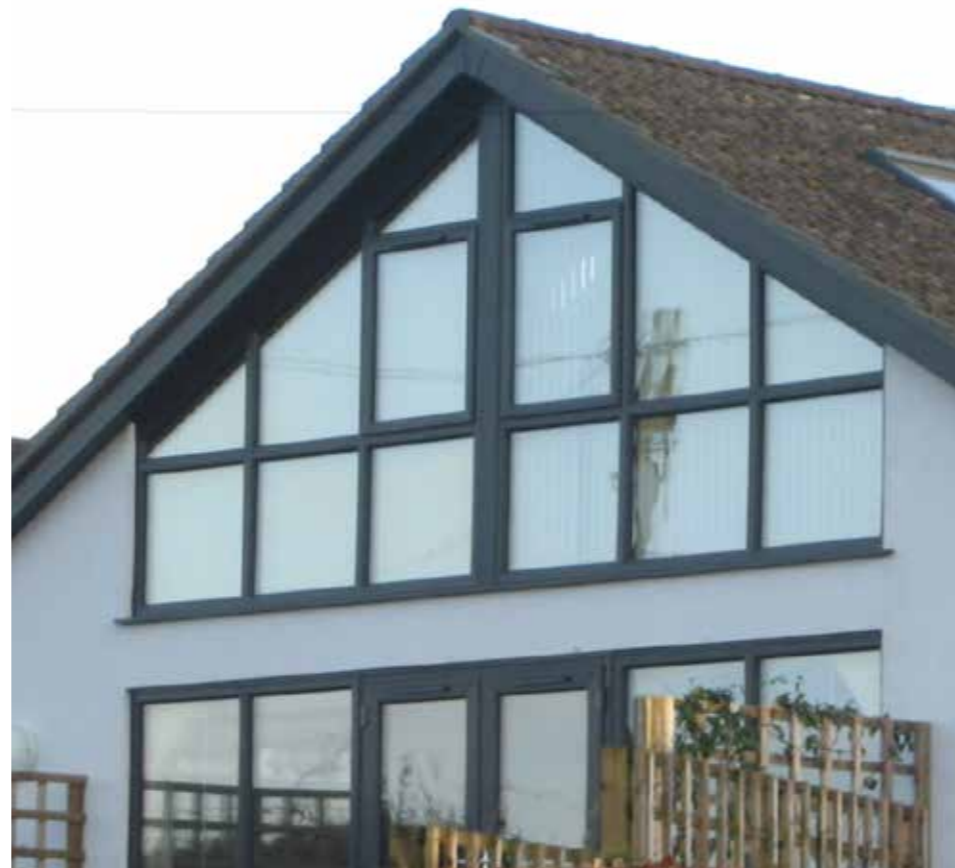
Different typologies of contemporary take on windows. Combination of fixed glass triple mirrored window, fitting the shape of the roof gable.
