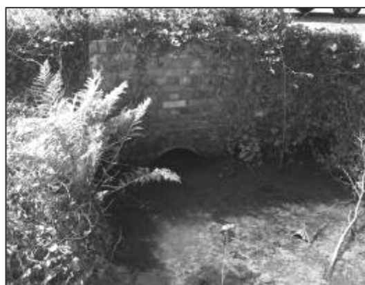
Figure 3.9 Structure 20 at Bournemouth airport – 100mm of silt and right hand pipe is partially blocked
