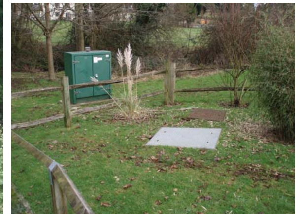
Small sewerage pumping station in Hawthorn Avenue
