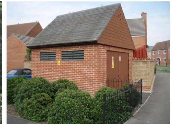
Electricity sub-station in Kingfisher Avenue
