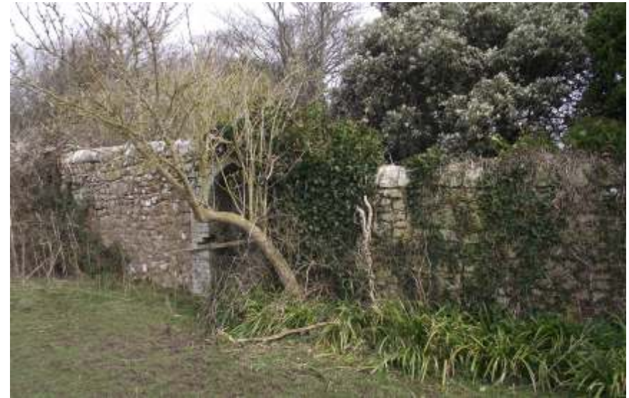
Plate 6 - Gateway in Wall to grounds of Nottingham House view south west to north east.
