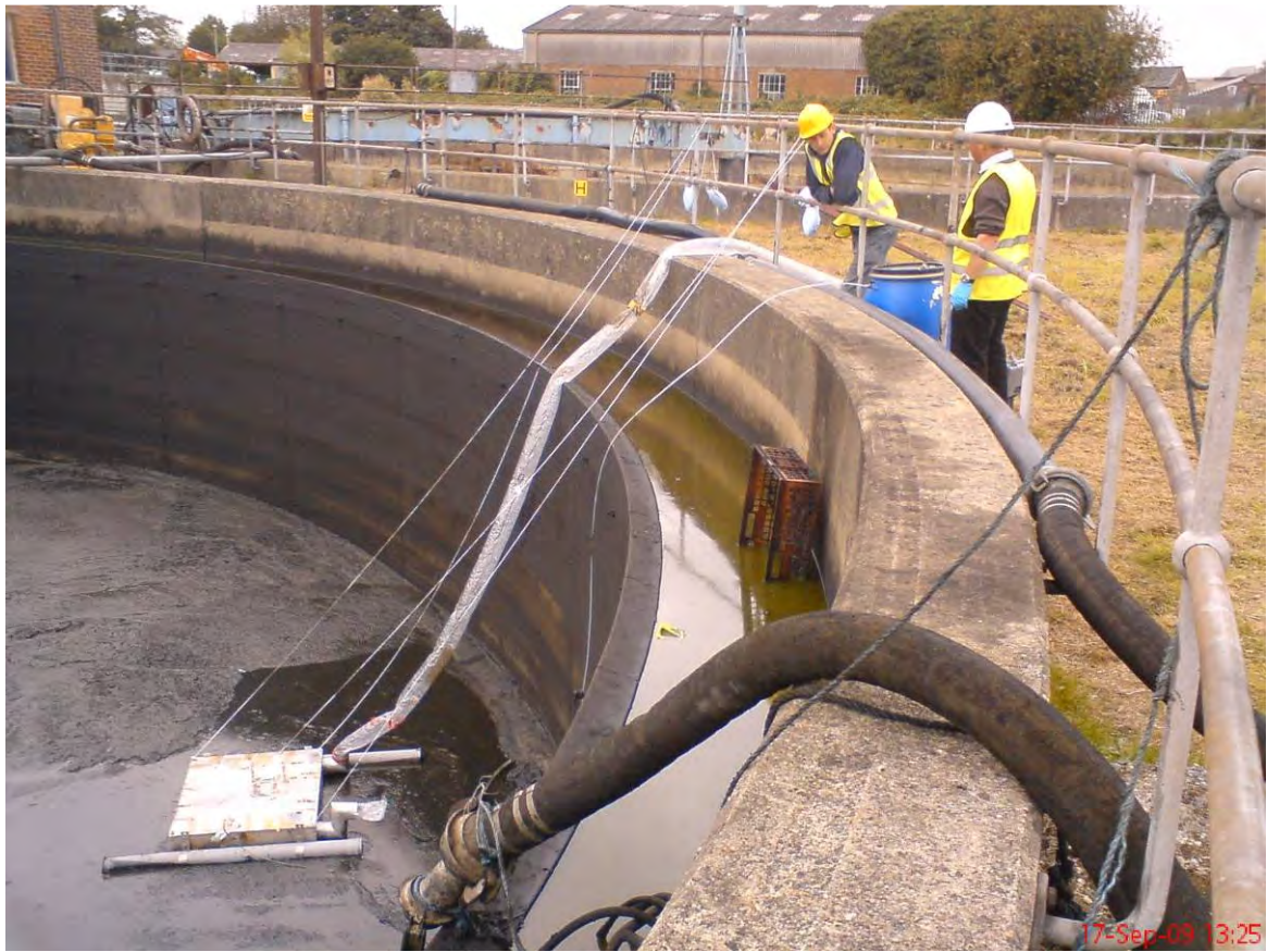
Fig 3, The Lindvall type hood collecting surface emissions from a sludge settlement tank.
