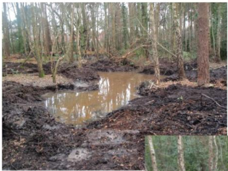
Feb/March 2009 Ponds are dug out to turn a widespread boggy area into a more defined and usable area.
