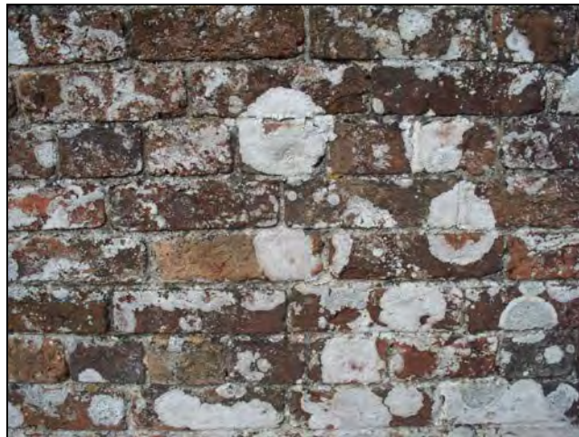
FIG. 16: Lichen on brickwork along Station Road.
