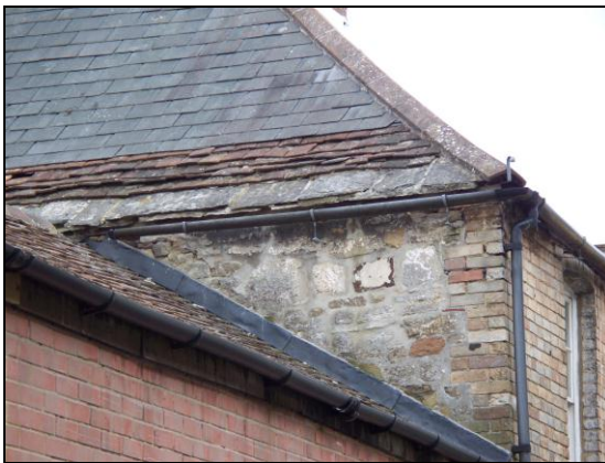
FIG. 16: Material palette. The rear of 8 West Street displays a range of materials and change over time. A fragment of the original tile covering with stone eaves course survives the rest replaced by slate. A bracketed gutter has been added. Whilst the frontage (FIG 8) is stuccoed, flank and rear walls reveal brick and stone construction which might suggest incorporation of older material within the post-fire rebuild.
