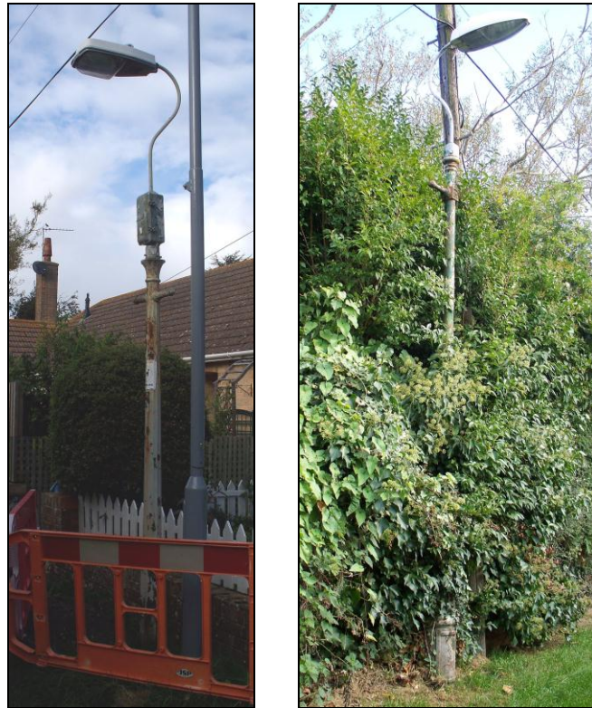
FIG. 13: Historic lamp columns. Currently in Tinker's Lane though soon to be removed.
