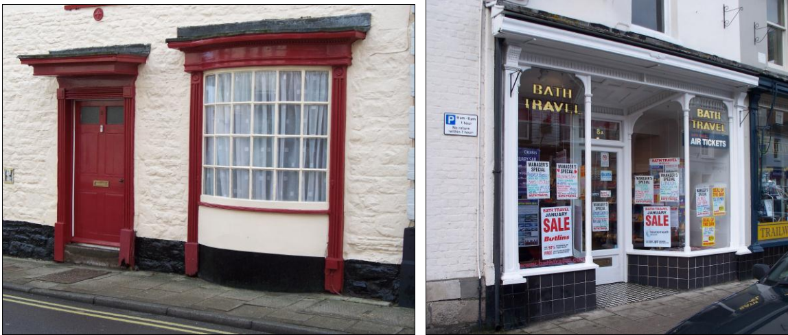
FIG. 18: Shop fronts. Left: early nineteenth century bow window serving a former shop at No 6 East Street. Right: Late nineteenth/early twentieth century shop front at No 8 South Street – note tiling and threshold mosaic.
