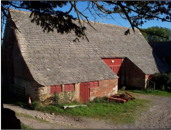
FIG. 10: Stone roofed barn. The barn is a prominent feature adjacent to the church opposite Church Farm Cottage.
