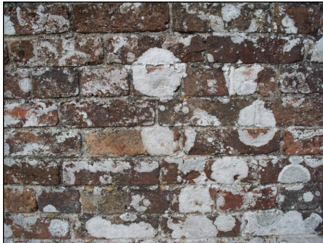
FIG. 17: Lichen on brickwork along Station Road.
