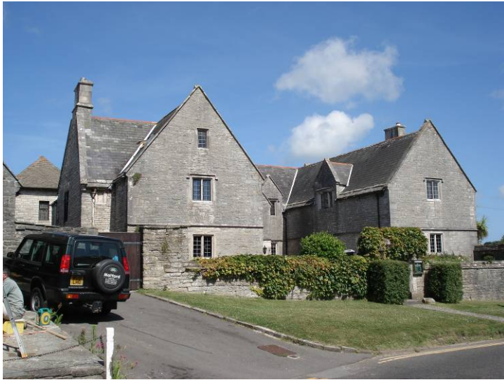
FIG. 2: Morton's House. The original parts of the building were constructed around 1600. It seems unlikely that slate was the original roof covering.
