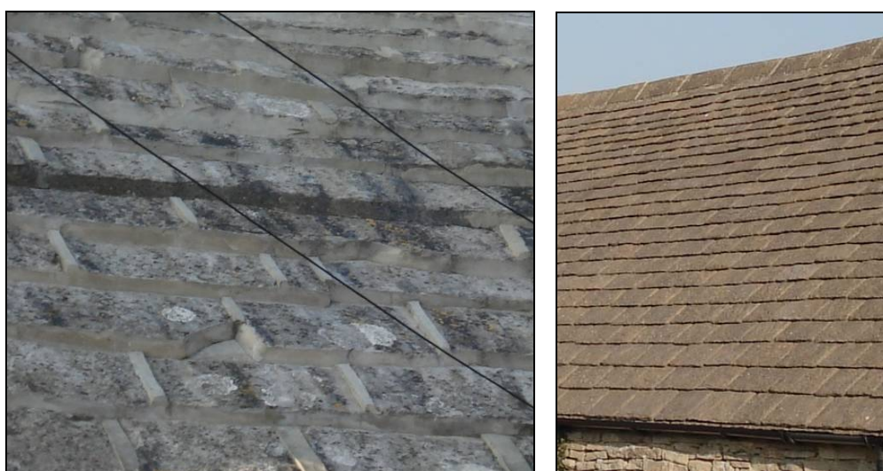
FIG. 9: Problems in roofing. Left: A heavily 'pointed' stone roof, now appearing more mortar than stone. Right: a modern synthetic stone roof with marked brownish colour which unlike Perbeck Stone will not weather to grey.
